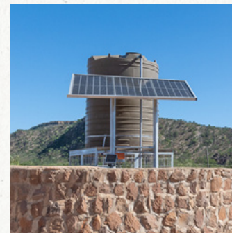
The upgraded solarized borehole in the Kunene Highlands, implemented by Conserve Global and funded by ECF. © Peter Chadwick.
